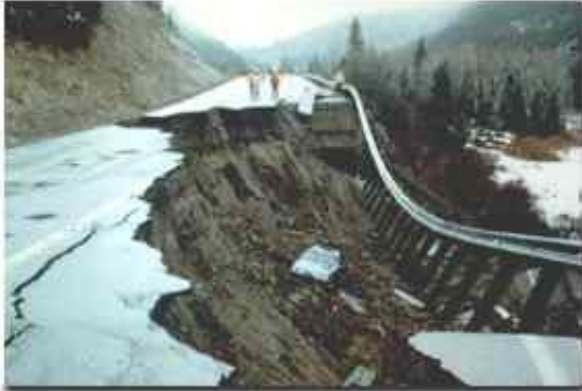
(Road failure caused by a landslide. Source of Photo: NOAA.)
